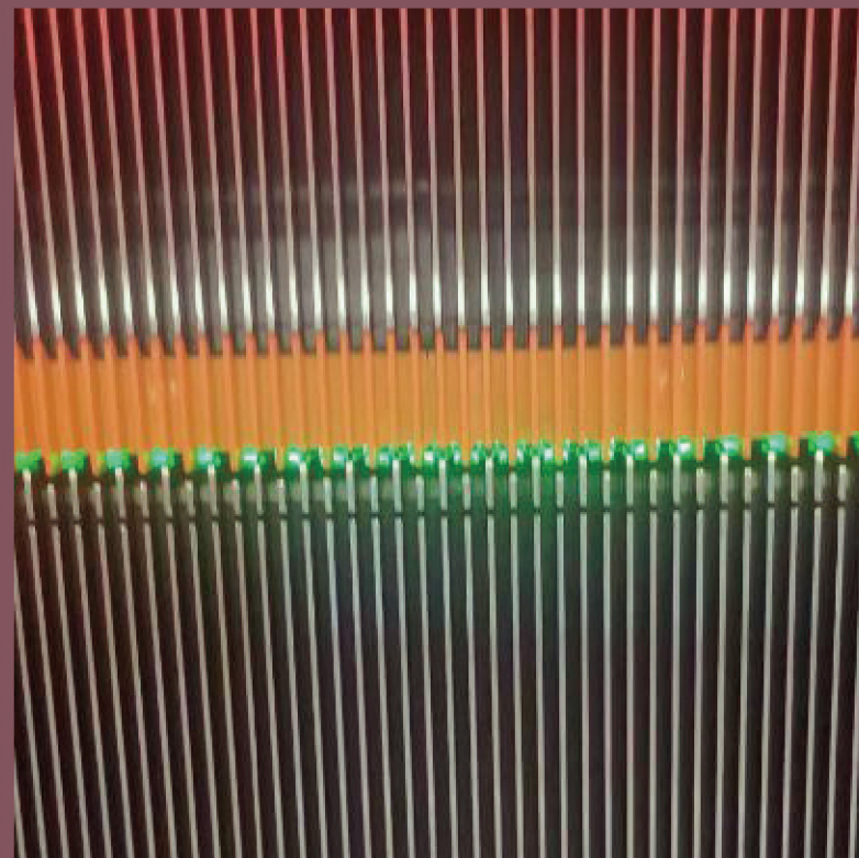
踏階下照明 Understep lighting
